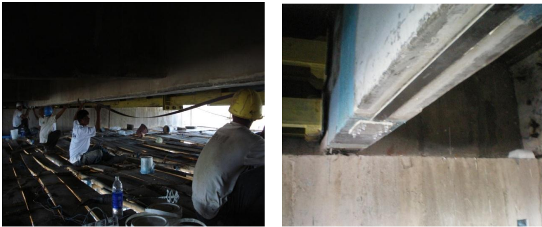
Figure 5. Pre-stressing in process and the finished laminate with anchor plates at end.
